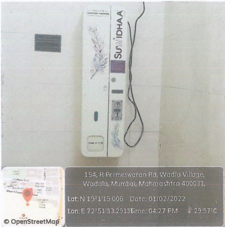
Sanitary pad vending machine in Ladies' washroom on third floor, Main building
