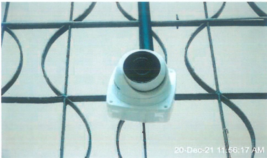
CCTV surveillance camera
