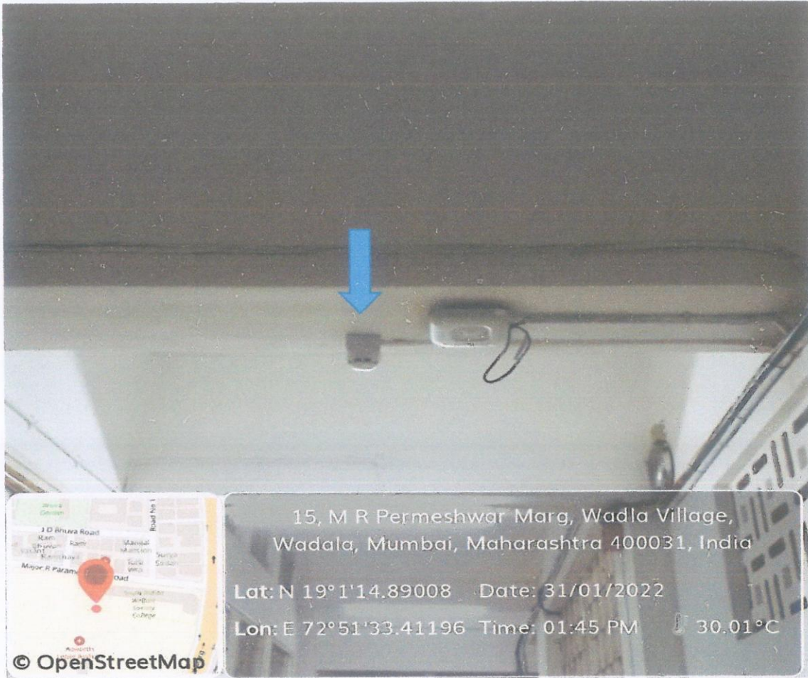
A smoke detector installed on the second floor, Central Building
