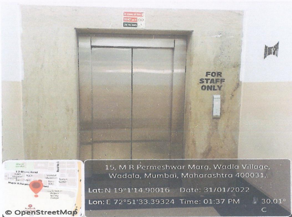
Sign Board above Lift Door 'Not to use lift in case of Fire'
