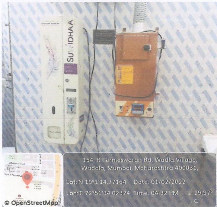
Sanitary pad vending machine and Incinerator in Ladies' washroom, Staff common room on first floor, Main building
