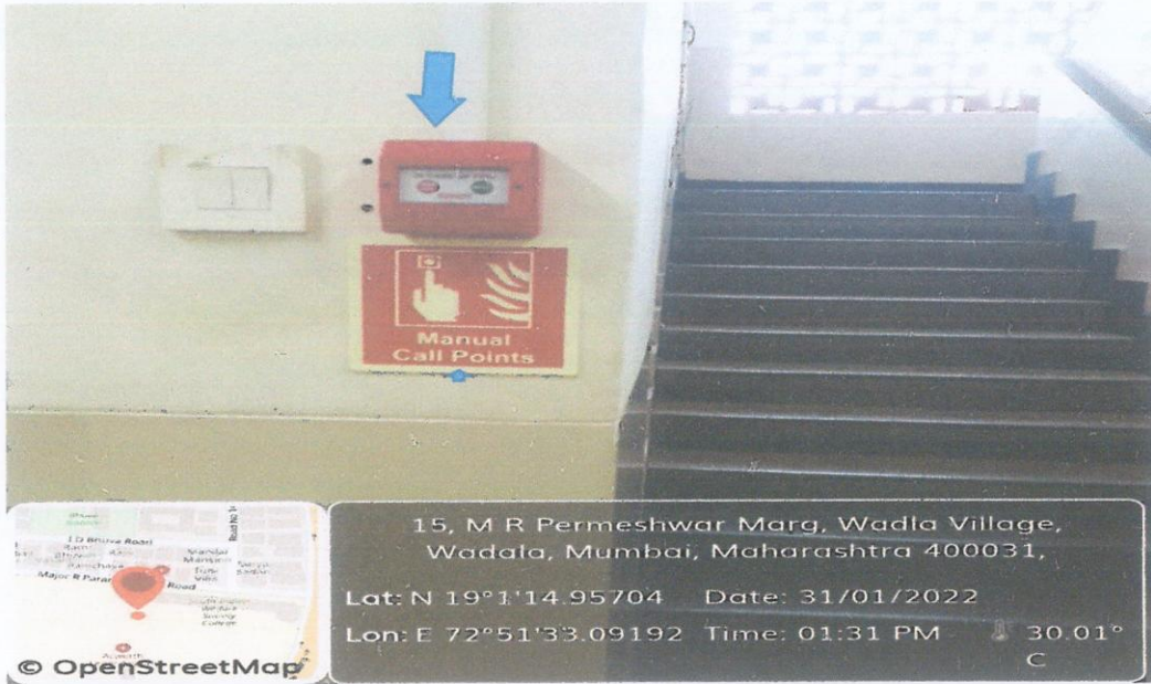
Fire safety alarm installed on the 3 rd Floor, Main Building
