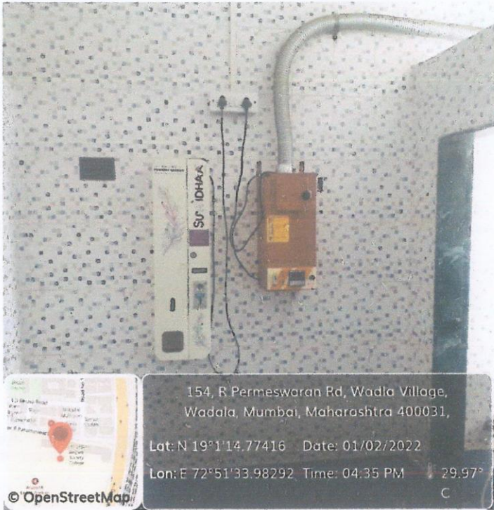
Sanitary pad vending machine and Incinerator in Ladies' washroom on first floor, Central building
