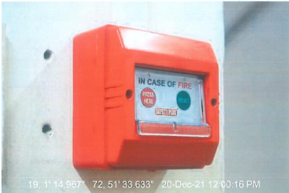
Fire Safety equipment
