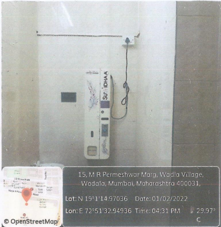
Sanitary pad vending machine on second floor, Main building
