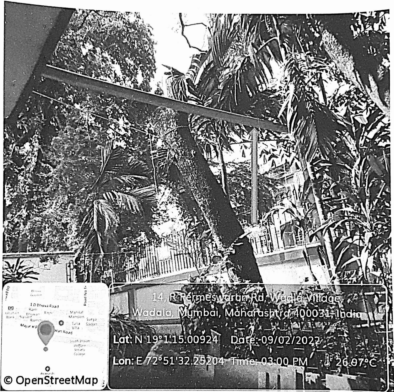
Pipeline carrying rain water from the terrace to the storage tank
