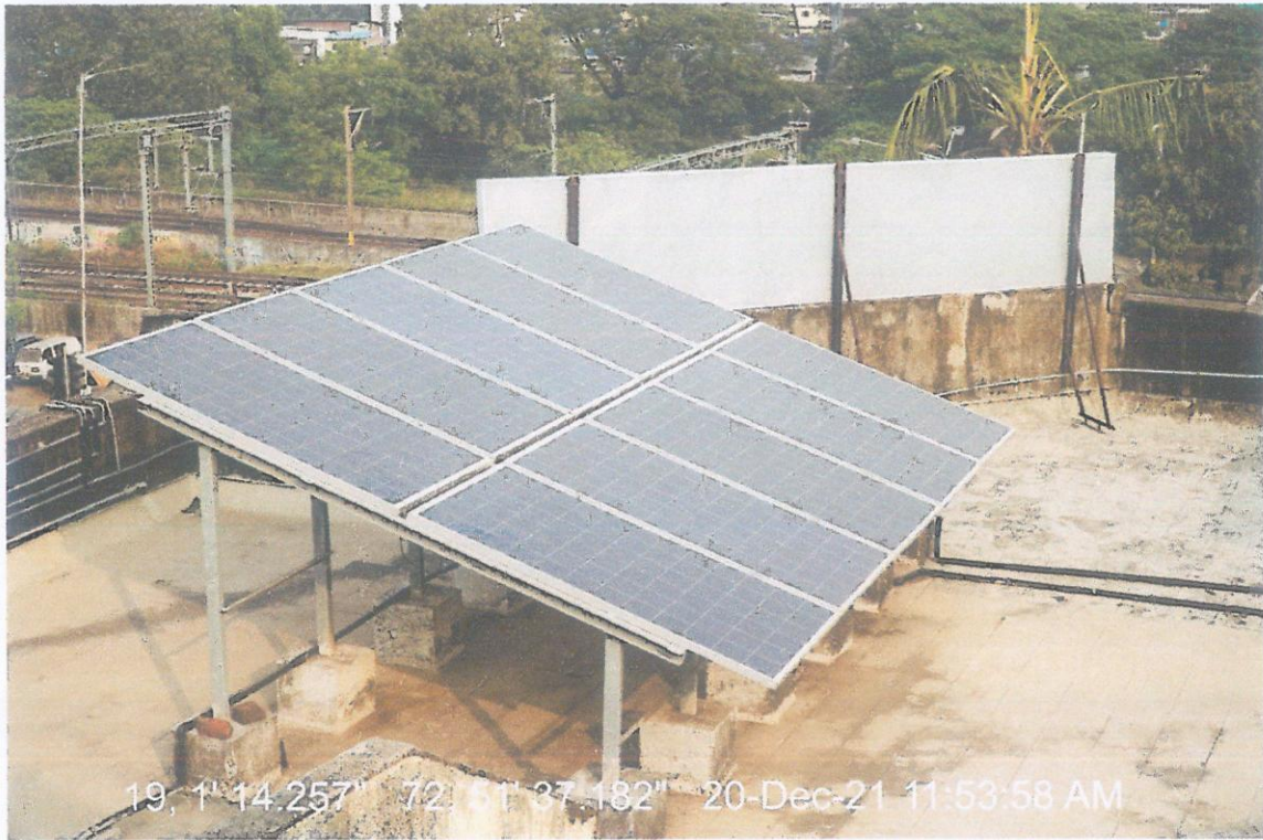
Solar Panels on the terrace
