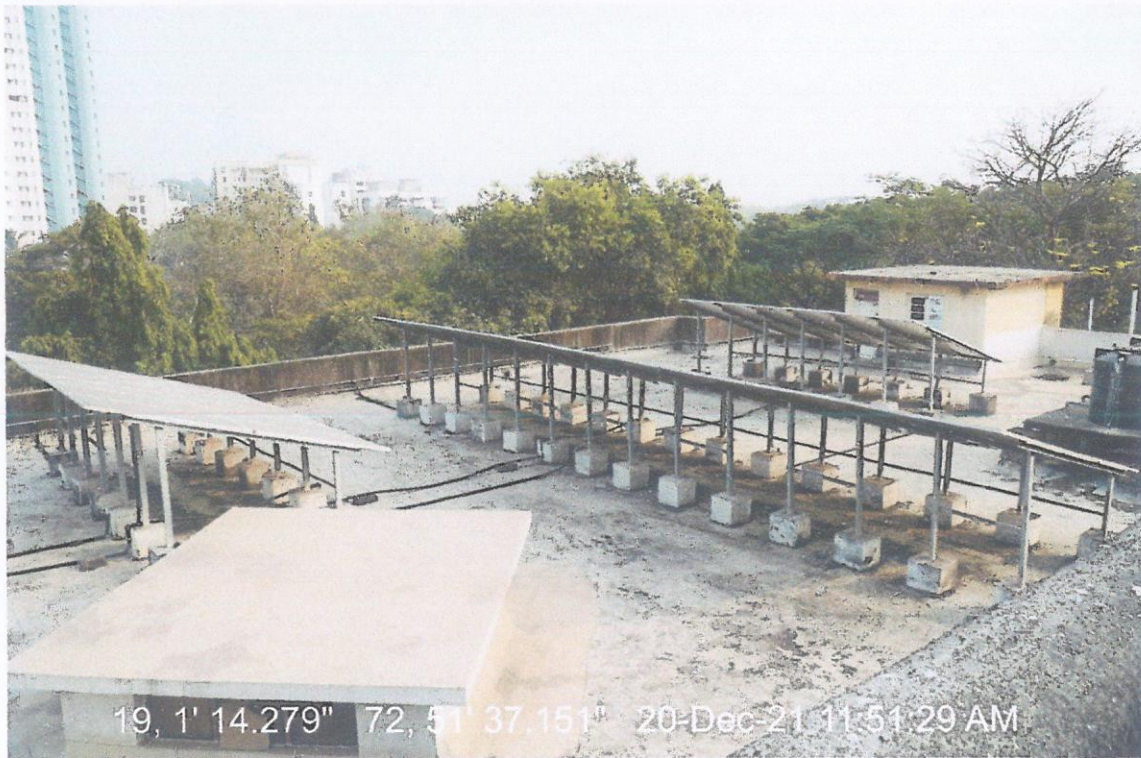
Solar Panels on the terrace
