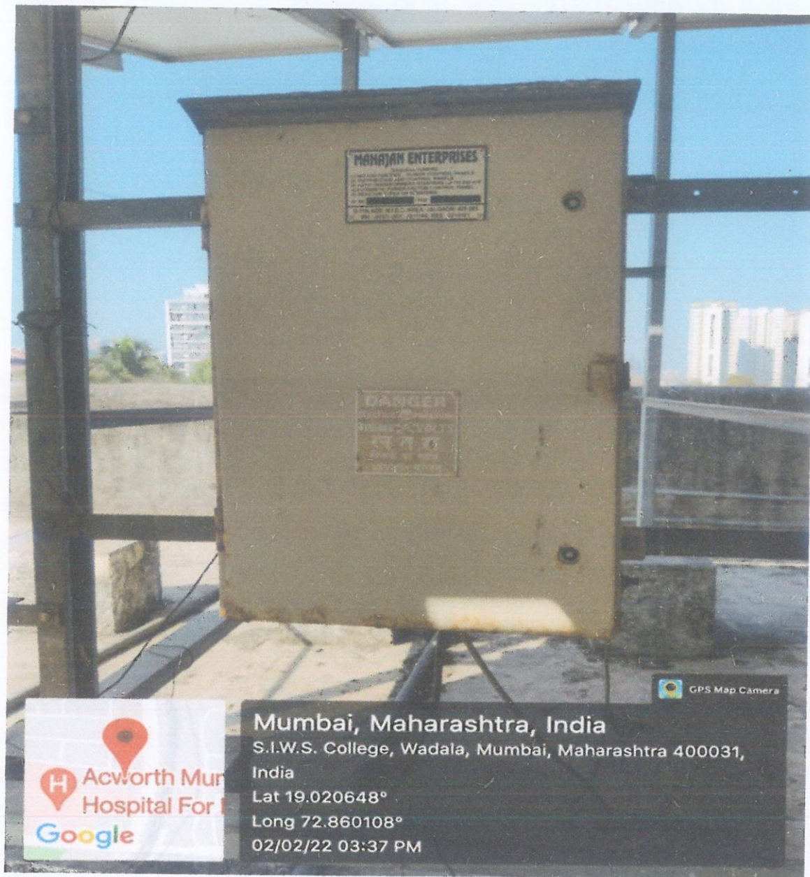
Inverter of Solar Panel
