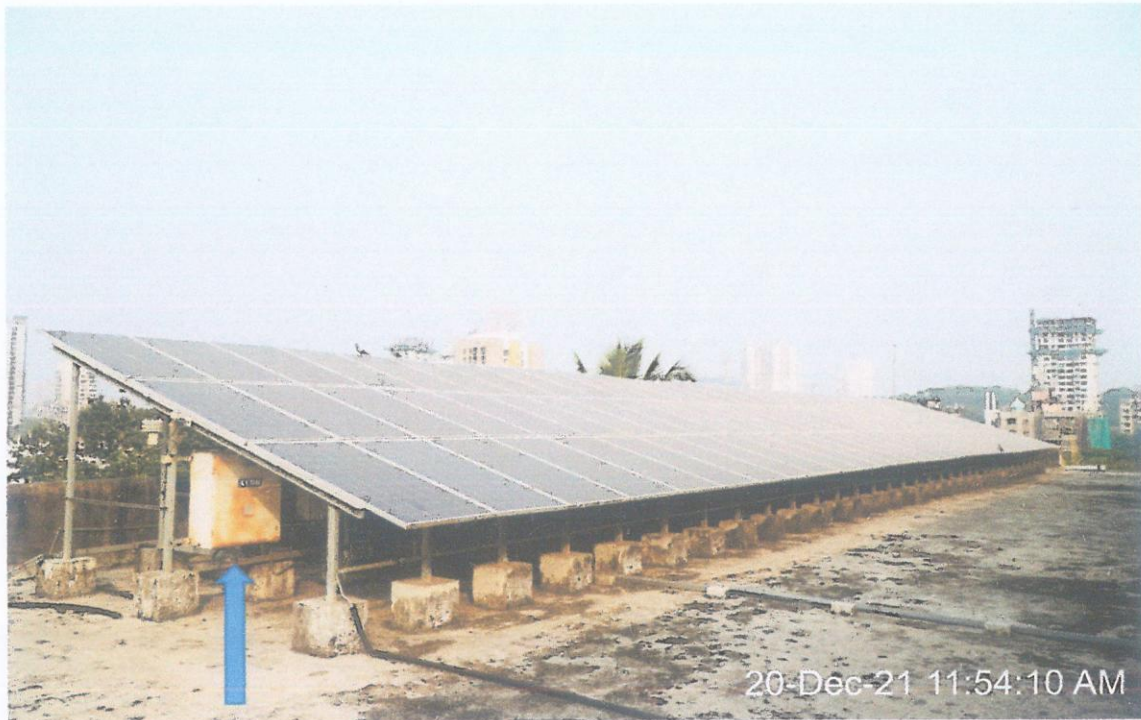
Solar Panel Inverter
