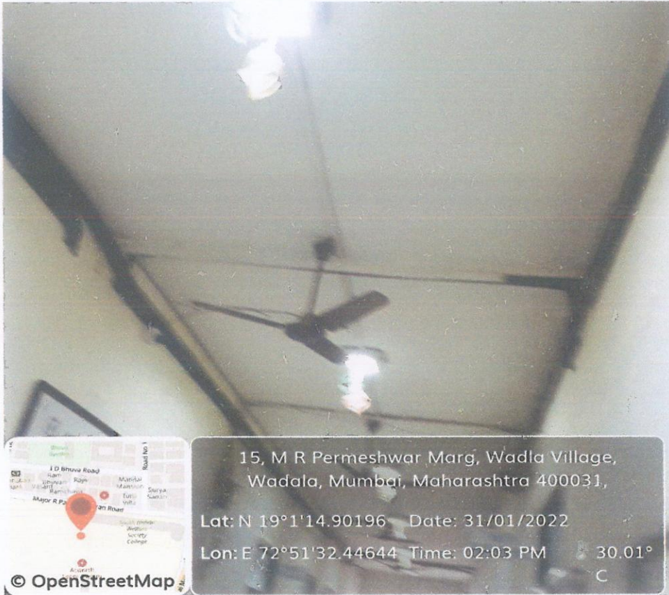
LED lights in the corridor, ground floor, outside the college office
