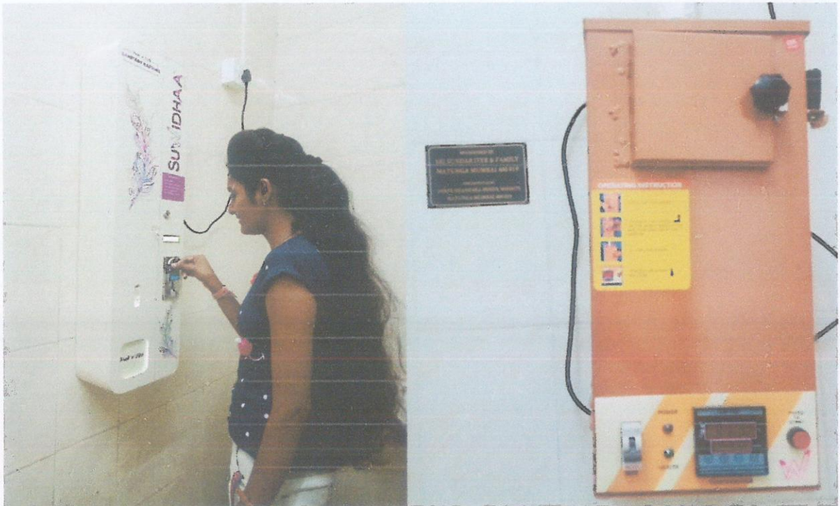
Student using the Napi Machine installed in Girl's washroom. (right side- incinerator)
