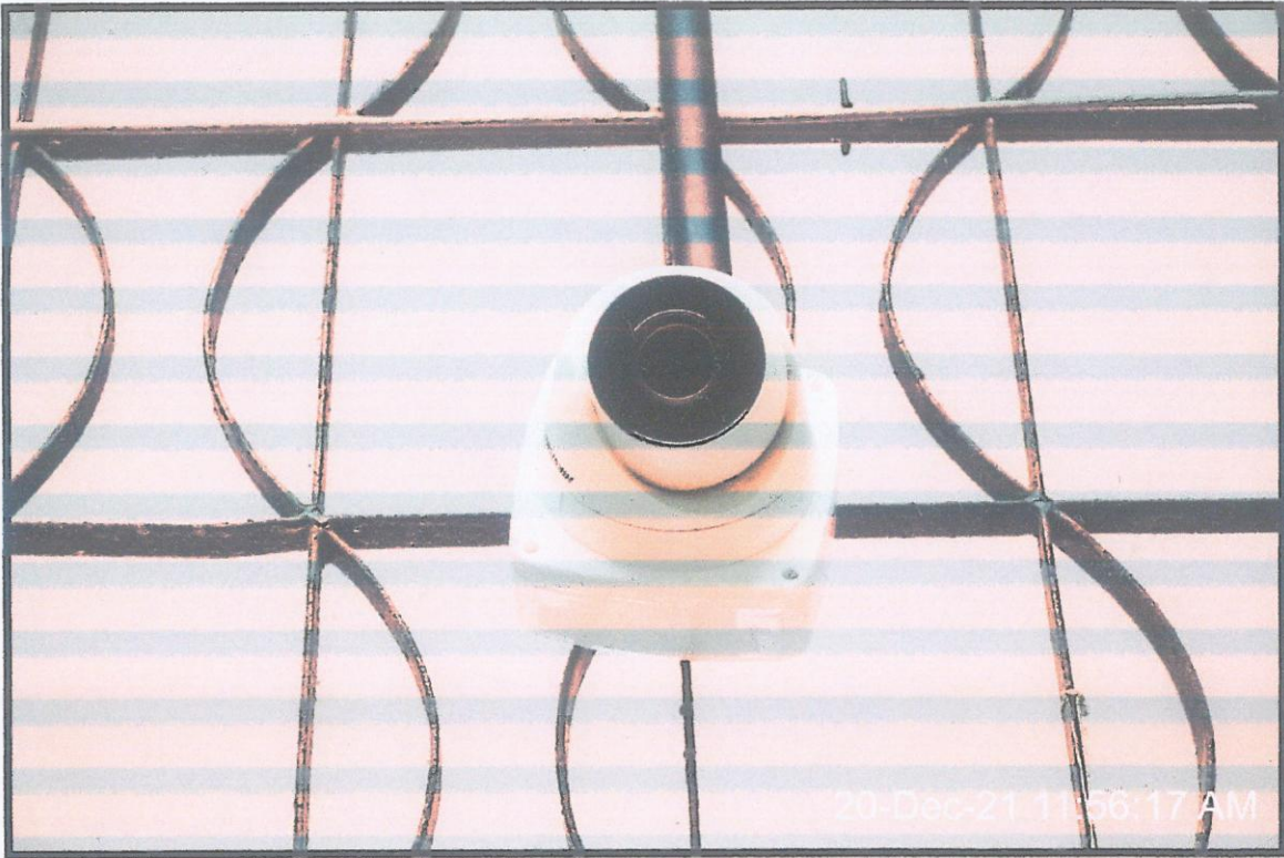
CCTV Camera installed in college campus at strategic locations for surveillance
